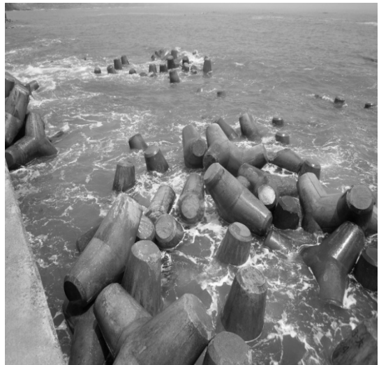
Fig.1 Damaged Sea-Block armour at Ooya Port
